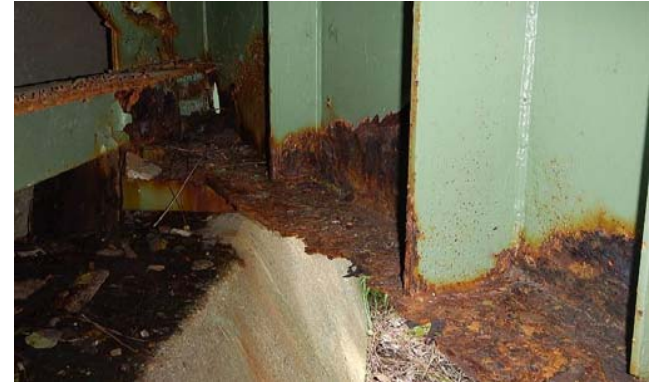
Poor (Structurally Deficient)
